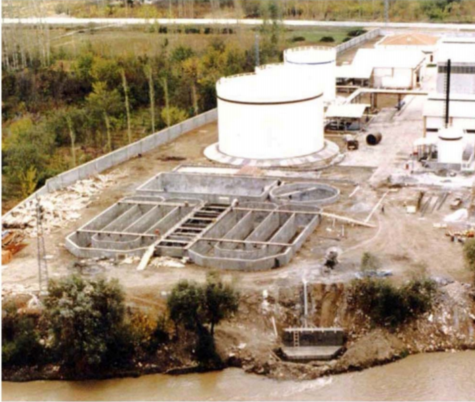
AMASYA SAFMAYA YEAST PLANT WASTEWATER TREATMENT PLANT (Phase 1)
