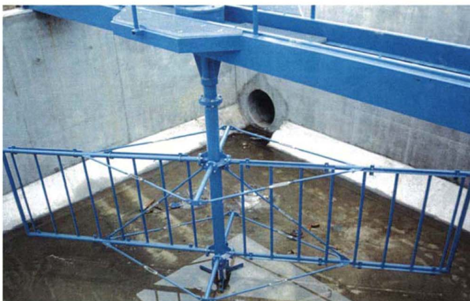
VERTICAL SHAFT PADDLE TYPE FLOCCULATOR
